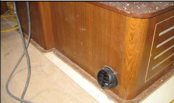
Runs outlet air duct from T junction inboard inside the bunk then install outlet nozzle on bunk lower corner.
