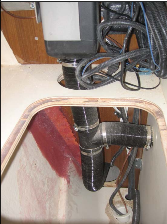
Air outlet locates underneath the heater unit. T junction under the heater distributes air to aft cabin and to main cabin.
