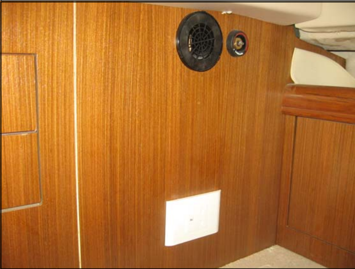
Drill \varnothing 1-3/8" hole on aft galley bulkhead for inlet air nozzle installation.
