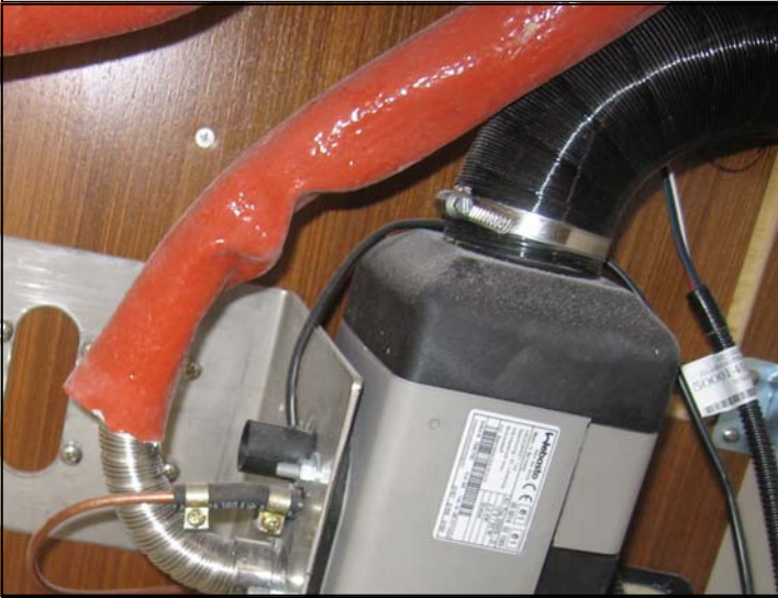
Heater inlet air duct facing upward. Inlet air vent locates on aft galley bulkhead
