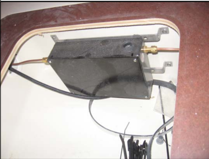
Fuel pump enclosure assembly locates under the aft cabin bunk port side forward face.
