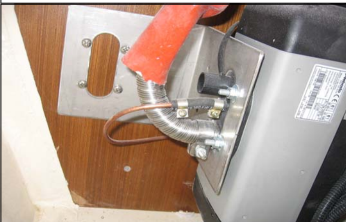
Heater exhaust tubing runs from the heater unit to outboard end. The fitting locates on port side sheer
