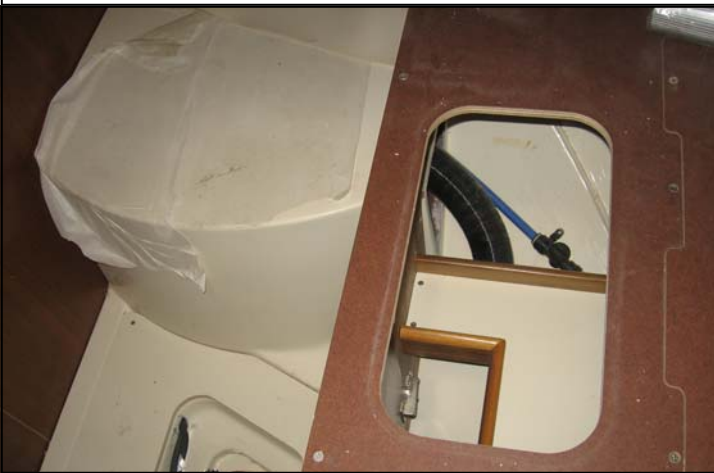
Air duct runs run through main bulkhead then inside V berth glass bunk then goes inside V berth bunk
