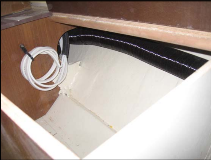
Air duct runs from T junction inside the bunk then going forward thru bunk divider.
