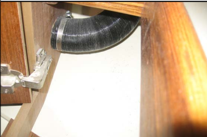
V berth outlet air duct is mounted and installed on air nozzle that mounts on bunk port side lower corner.
