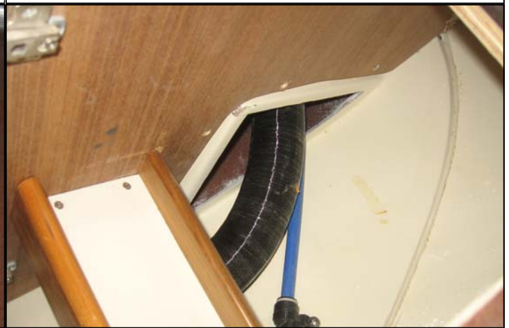
Air duct comes out V berth glass bunk then goes under the shelf
