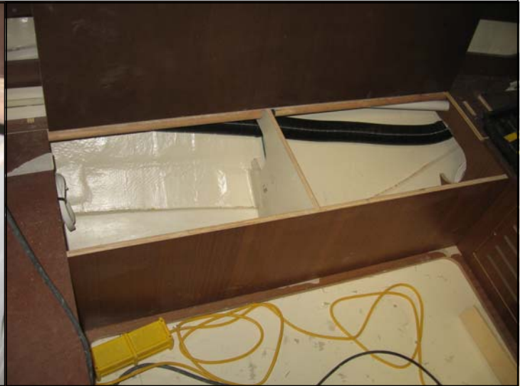
Air duct runs inside the bunk then going forward thru bunk divider then thru main bulkhead.
