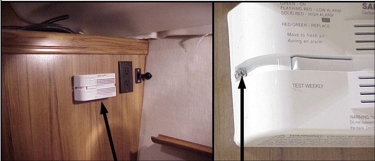
CO MONITOR ON Q-BERTH HANGING LOCKER
