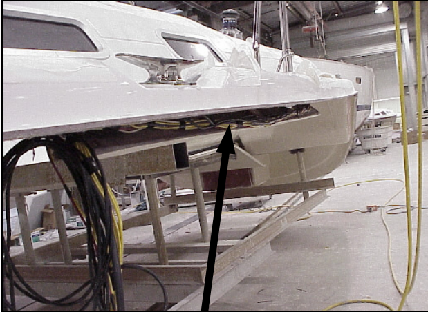
WIRES RUNNING AFT ALONG TOP OF HEADLINER
