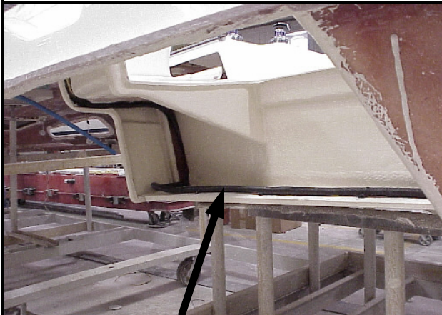
WIRES RUNNING AFT ALONG BOTTOM OF COCKPIT WALL
