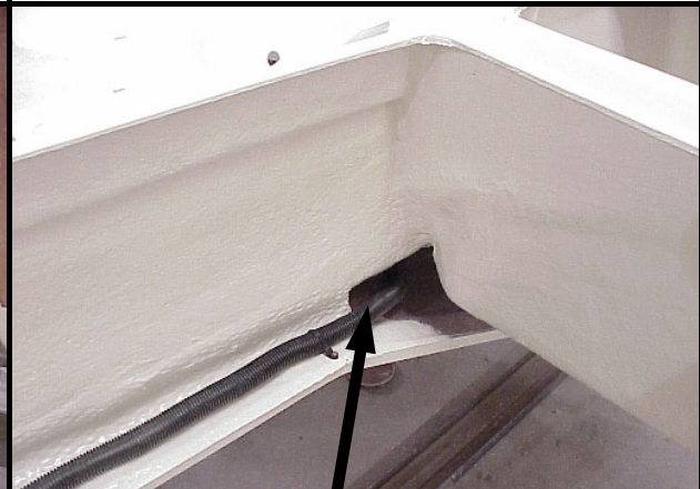
WIRES RUNNING INTO AFT END OF HEADLINER
