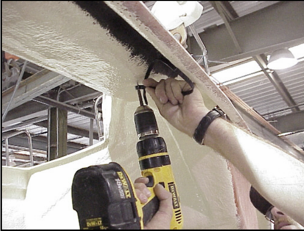
ATTACH AFT CABLE TIE TO UNDERSIDE OF DECK APPROXIMATELY 18" FORWARD OF AFT WALL IN THE LAZZERETTE COMPARTMENT
