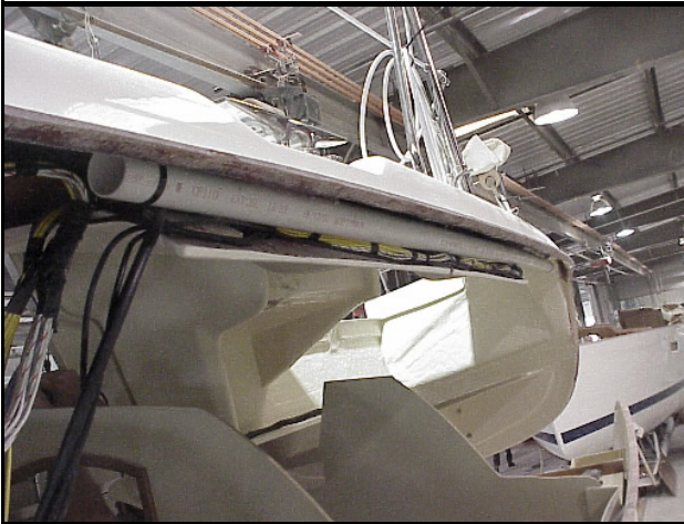
PICTURE OF TUBE RUNNING DOWN UNDERNEATH THE PORTSIDE OF THE DECK. SHORE POWER, 110 VOLT, AND SPEED & DEPTH CABLES WILL RUN THRU THIS CHASE TUBE
