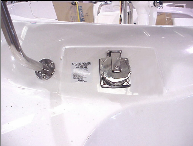
SHORE POWER OUTLET IN PORT- AFT CORNER OF THE DECK
