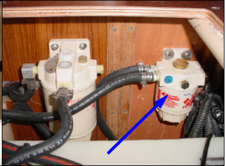
Mount generator Fuel filter next to engine fuel filter.
