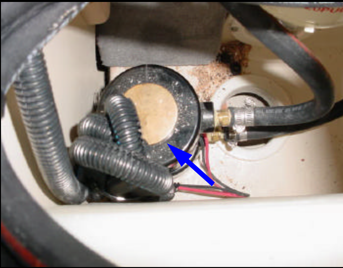
Generator fuel pump locates under fuel filter.
