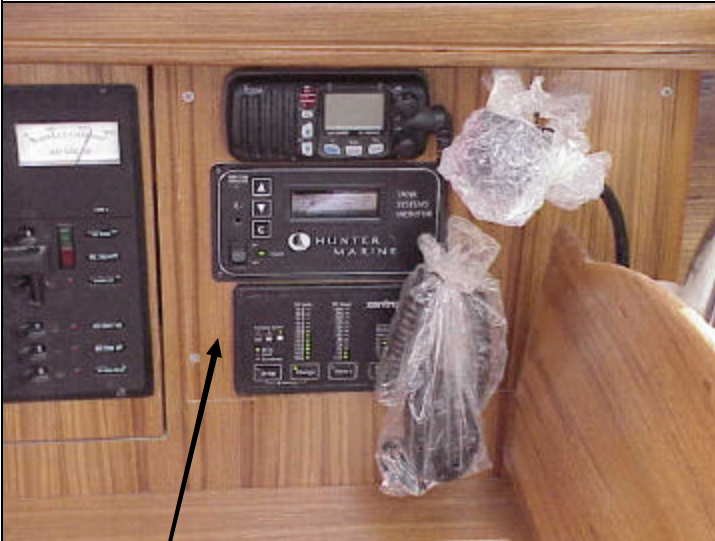
Course computer located in forward end of nav station. Access is gained by removing front face of nav station.
