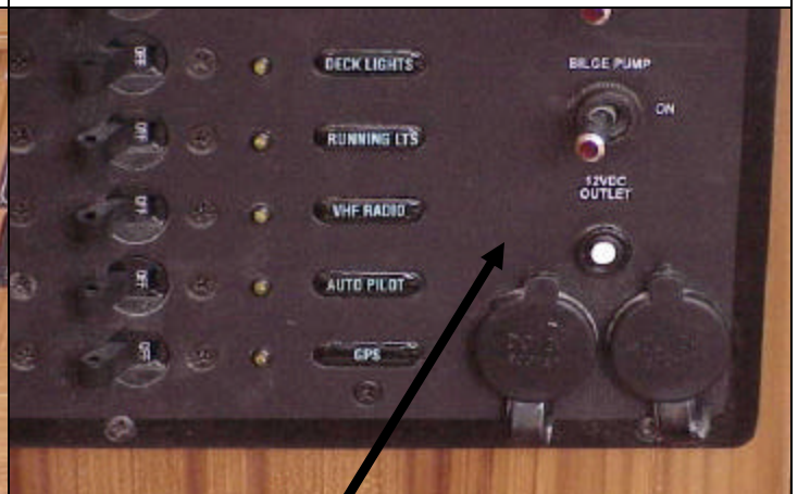
The spare "Instrument" breaker will need to be removed and replaced with a 25 amp breaker for the auto-pilot.
