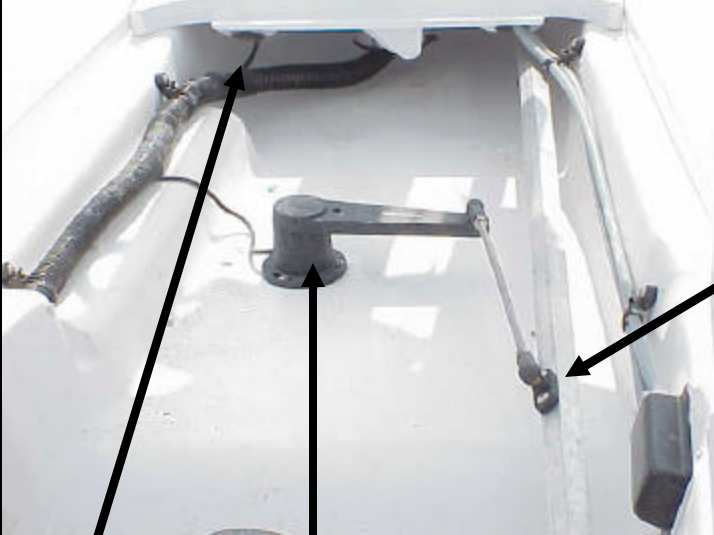
Rudder reference sensor unit attached to deck with rudder sensor unit tie rod attach to unit and pivot ball. Notice wire from sensor unit going up port tube of steering pedestal grabrail.
