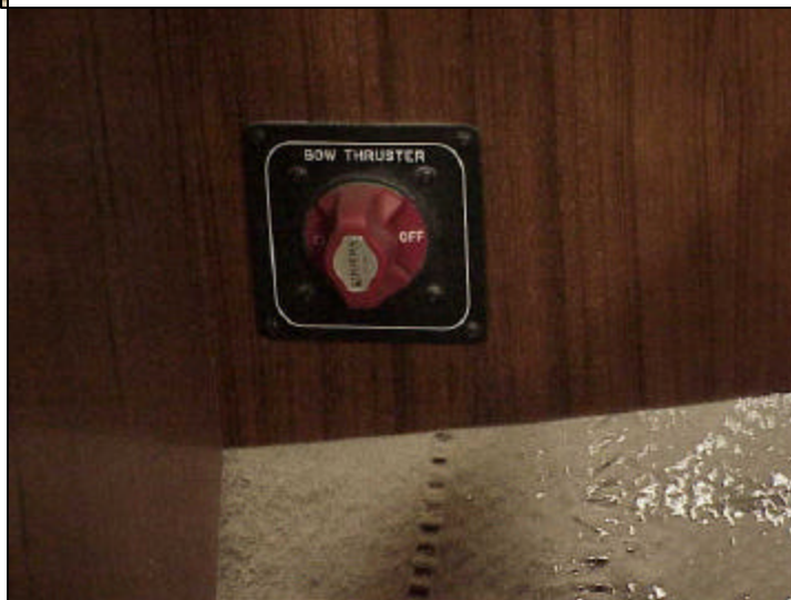
Location of isolator switch that will need to be installed on outboard face forward of nav seat.
