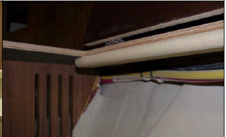
Cables continuing under the bunk top, the PVC pipe.
