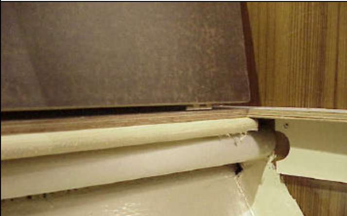
Cables continuing thru PVC pipe under the bunk top, the PVC pipe only runs halfway under the bunk.
