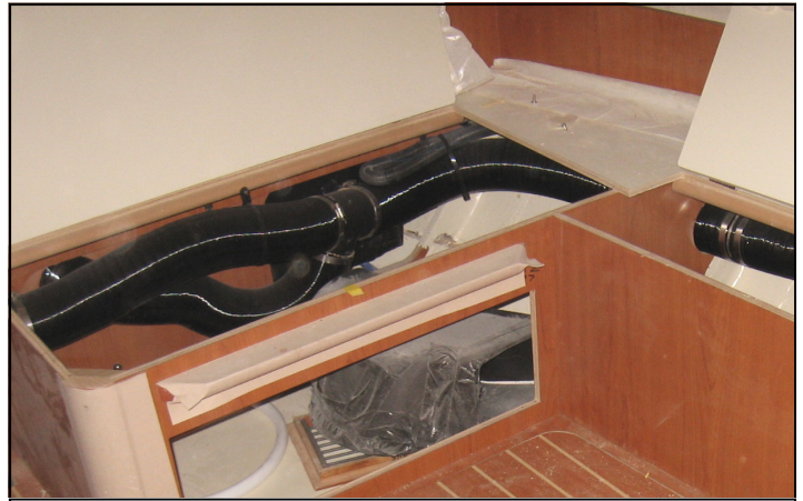
The picture shows ø3.54" ducting layout locates in fwd bunk which distributed for main cabin and V berth cabin.
