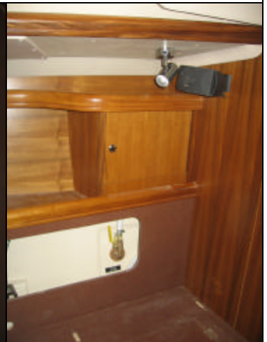
Fwd AC discharge thru hull ball valve
