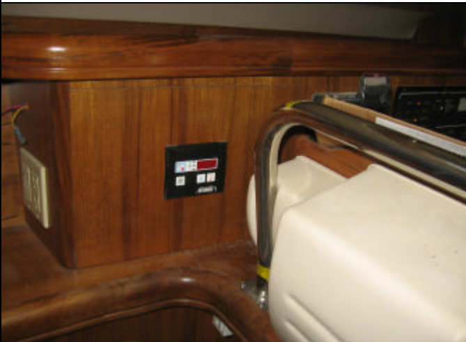
Main Cabin Air Cond Control locates at fwd corner of the electrical panel by NAV station.
