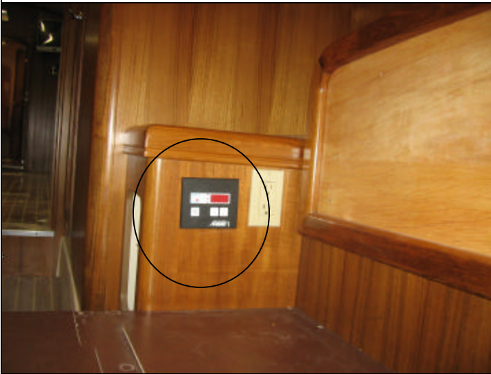
Aft Cabin Air Cond Control Location
