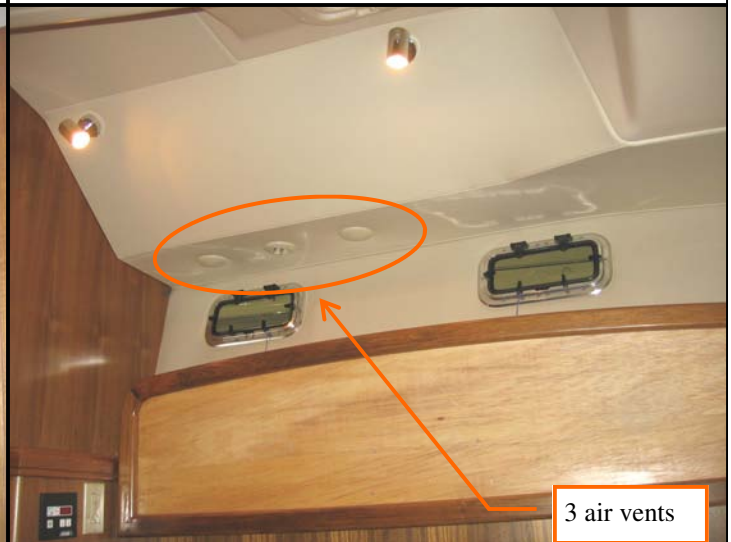
3 air vents locate above aft cabin starboard side forward portlight area
