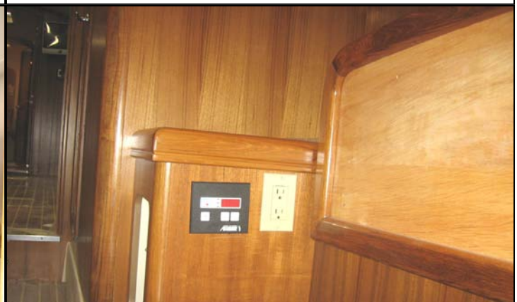
Aft air cond control panel locates on aft cabin starboard storage cabinet by 110V/220V outlet.
