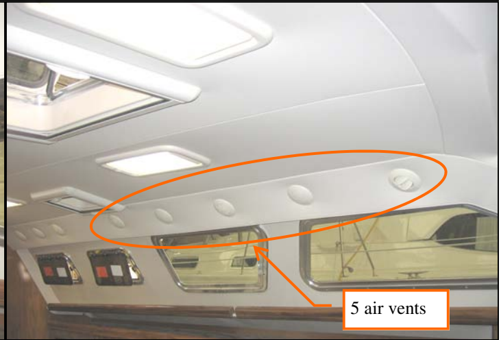
5 air vents locate above main cabin port side deck window area.
