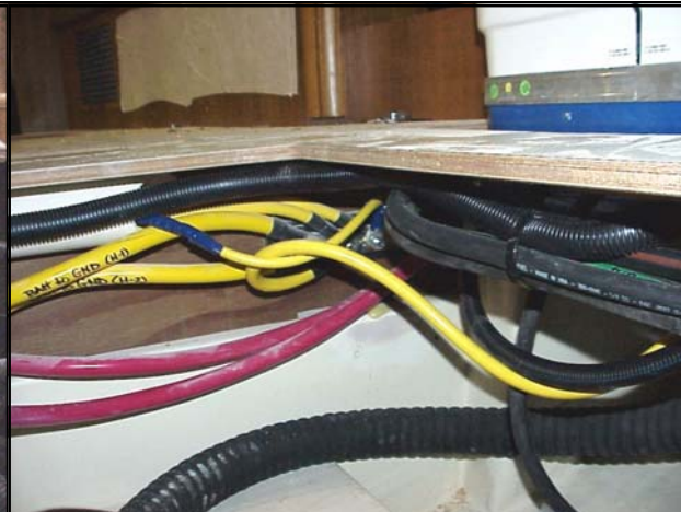
Ground cable (#10) running forward and attached to the ground buss bar on the wood stringer under the sub-floor.
