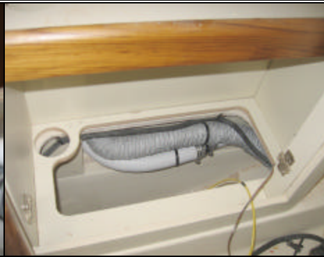
Inside fwd vanity lower cabinet, tie wrap air duct with waste feed hose inside lower vanity cabinet.
