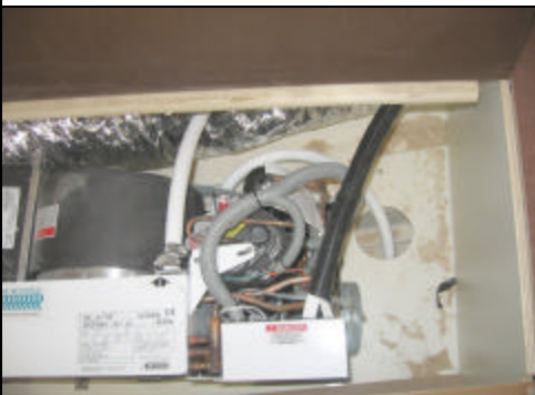
run this air duct from distribution box afterward, thru bunk divider cutout to aft bunk compartment
