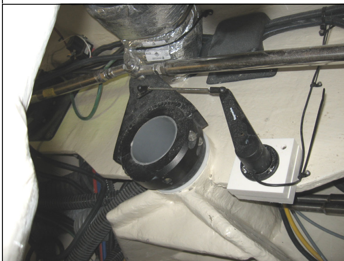
Autopilot rudder reference locates next to rudder quadrant
