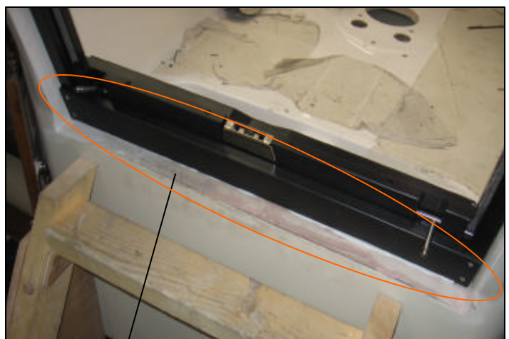
Overview from inside lower, the the gap has been closed by sealant
