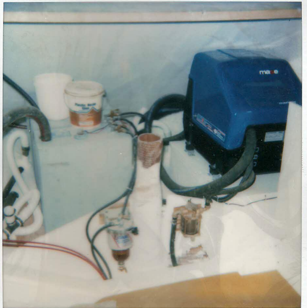
FUEL TANK + FILTERS GEN. GENERATOR H-45
