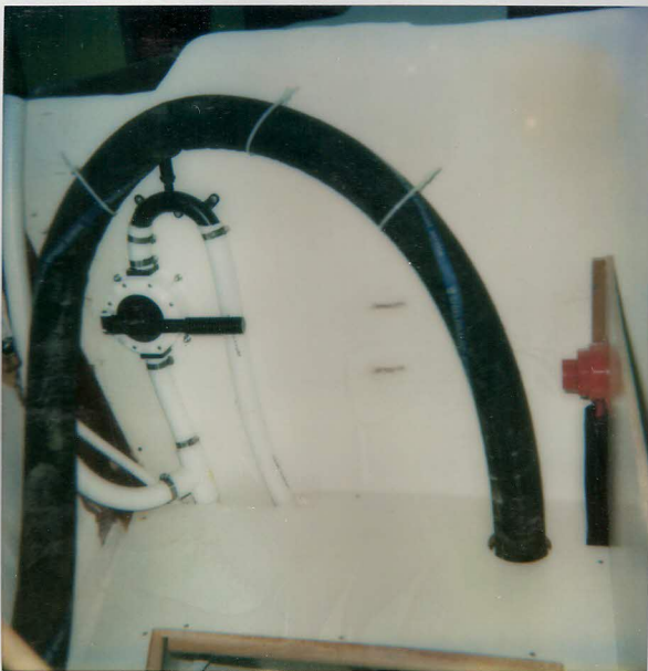
PORT AHA Pump out H-45
