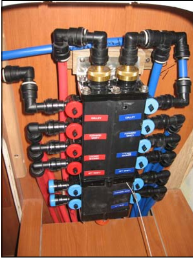
The picture shows waterline arrangement the old fresh water manifold before replacement
